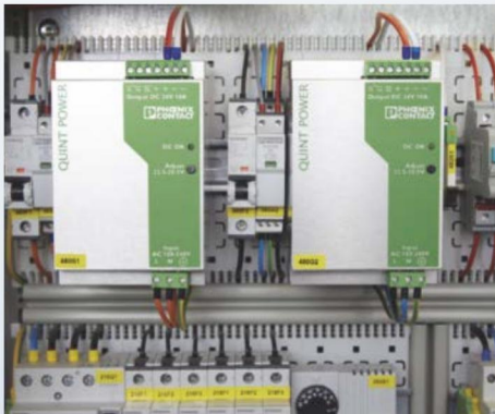
Power supply protection
